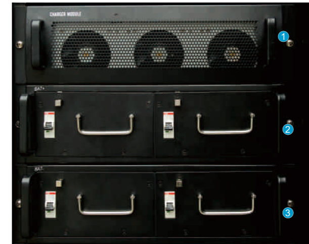
System front view
